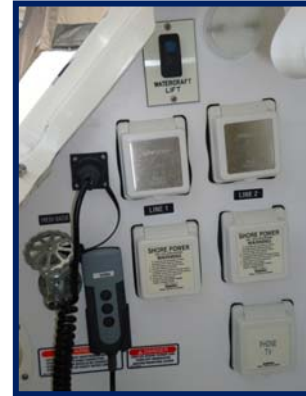
Shore Power Connections
